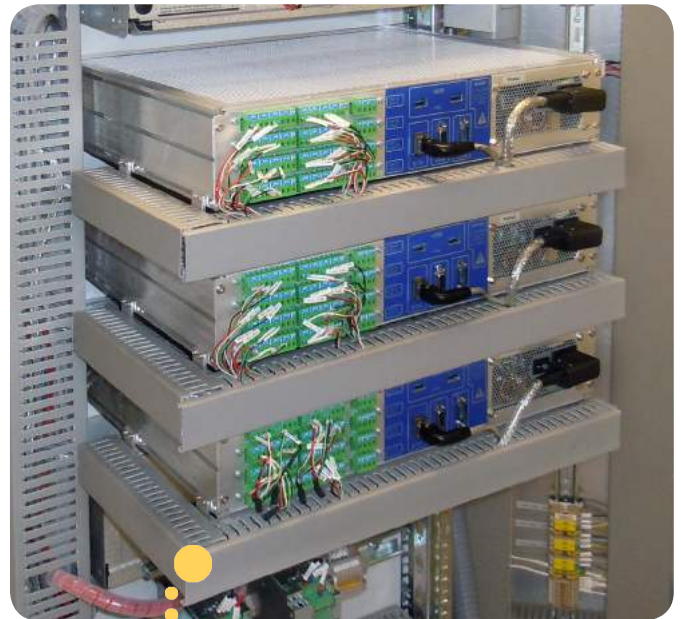
View from the back - connection of units
